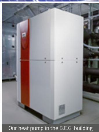
Our heat pump in the B.E.G. building
